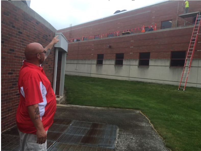
Figure 4: Steven Daniel Walden pointing at a new PVC roof that was just installed
